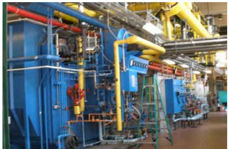
Farmingdale College - Central Utility Plant
