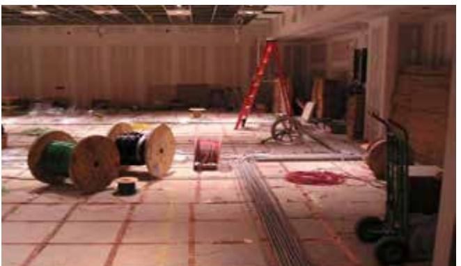
Command and Control Facilities
