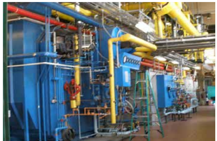
Farmingdale College - Central Utility Plant
